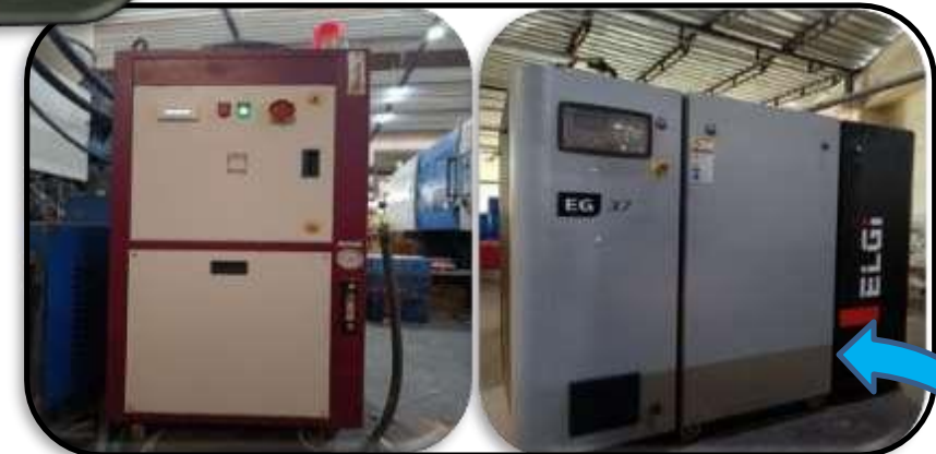
Water chiller and Compressor with VFD
